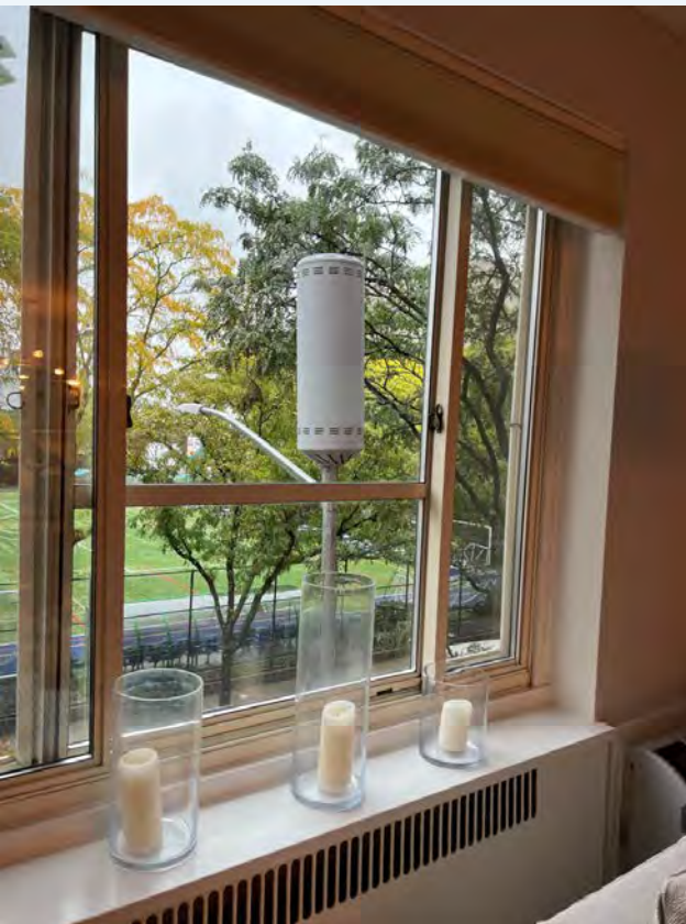
New York City "small cell" antennas in front of living room window.
